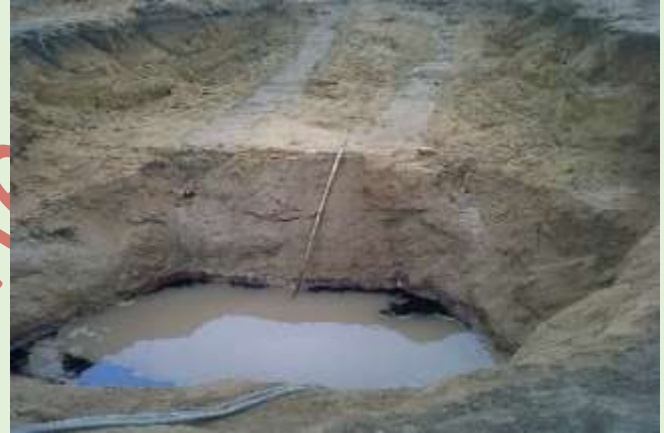
Groundwater condition in excavated pit after recovery and application of OSE II
