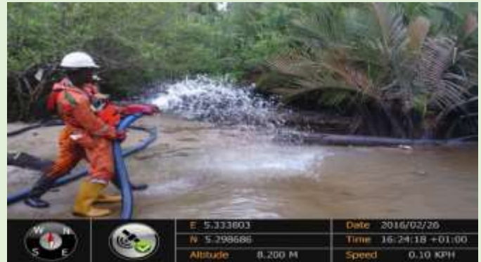
Fig 6: Flushing along the beach
