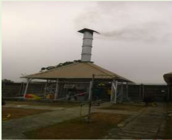
CNL Medical Waste Incinerator, Warri
